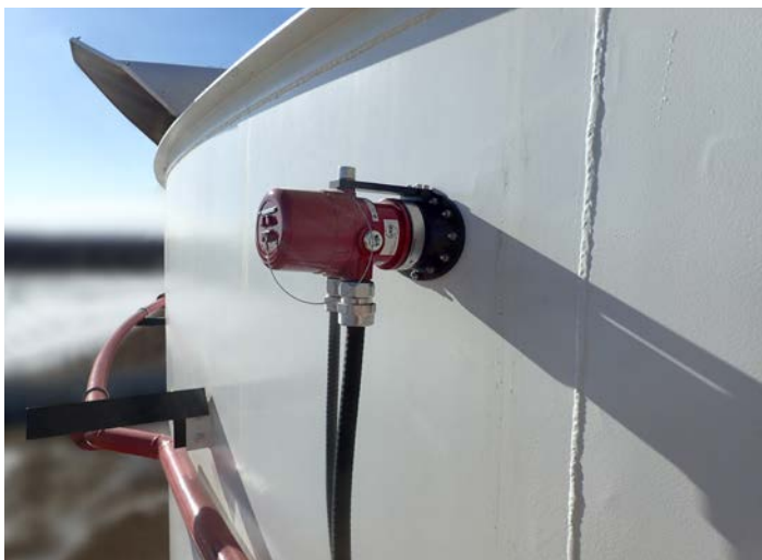
In this Zone 1 classified fixed-roof internal floating tank application, the optical flame detector is flange mounted. This installation technique allows for easier maintenance of the detector.
